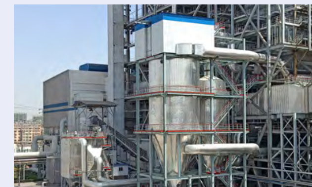
"Bypass Flue Gas Evaporation and Drying of Desulfurization Waste Water" demonstration project of Huangtai Power Plant
