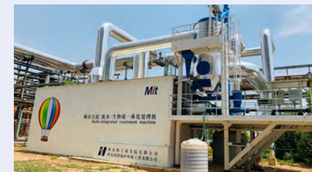
The "Key Technologies for Urban Waste Drying and Carbonization Pre-treatment" Demonstration Platform of Yueyang Power Plant
