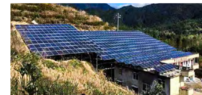
Distributed Photovoltaic Power Station in Shangyang Village, Dehua County
